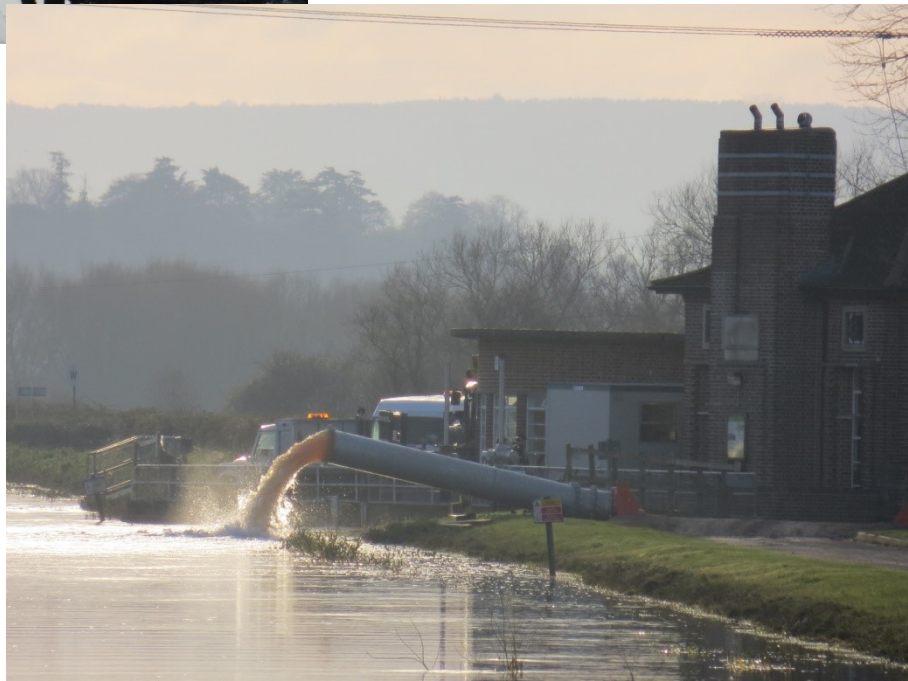
Currymoor pumping station with additional pumps
